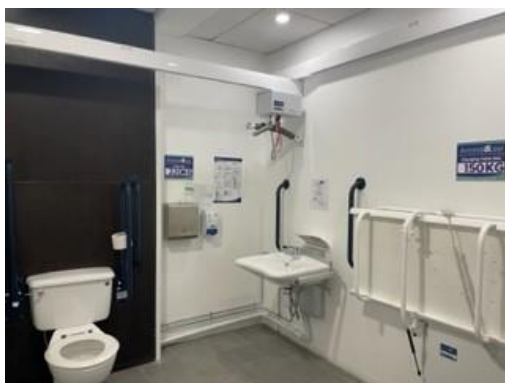
Figure 7: Changing Places toilet
